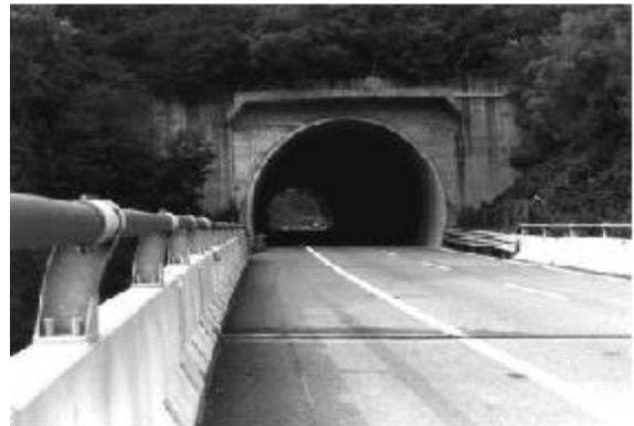
Fig. 3. The Uvi Tunnel portal (Torino side, Turin–Savona motorway). It is made of concrete and appears to be a solid structure with linear frontal and lateral walls, refined by functional wall brackets, which protrude above the inlet.
