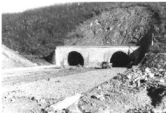
Fig. 2. Casarza tunnel, on the Milan–Rome motorway. The slope-supporting wall is a blot on the whole landscape and a remarkable amount of ground stripping is evident.
